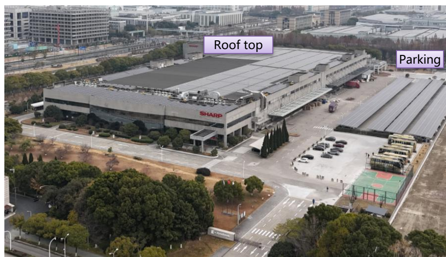
Solar power generation equipment
